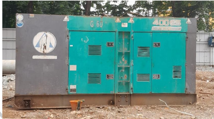
Gambar 3. 18 Generator Set Diesel
