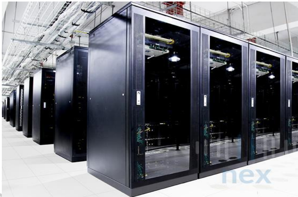
Gambar 2. 3 NEX Datacenter PT Cyberindo Aditama
