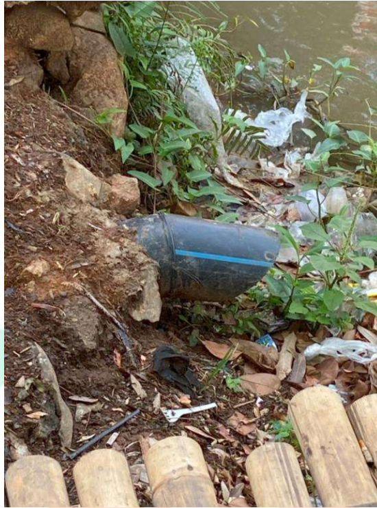
Gambar 4. 16 Aktual Pipa Washout
