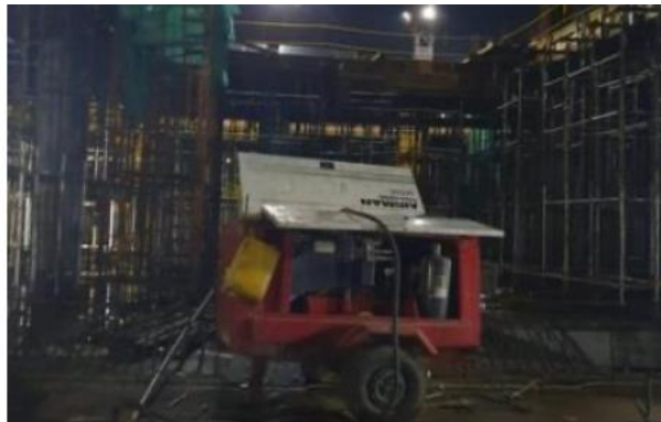
Gambar 0.20 Air Compressor Merk Airman
