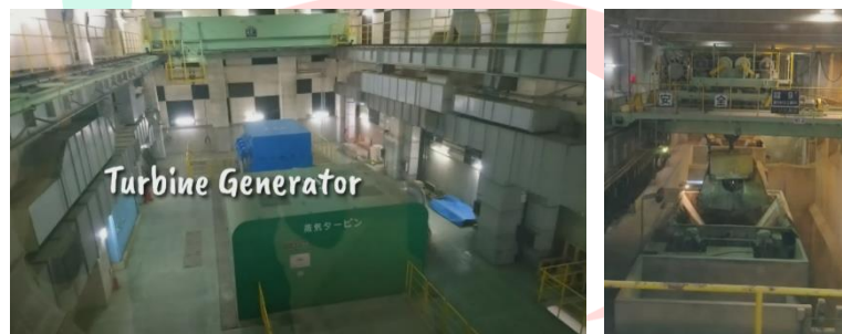
Gambar 2. 15 Ruang Generator Maishima Sumber: https://youtu.be/FDNcahZcG_Y , 2022
