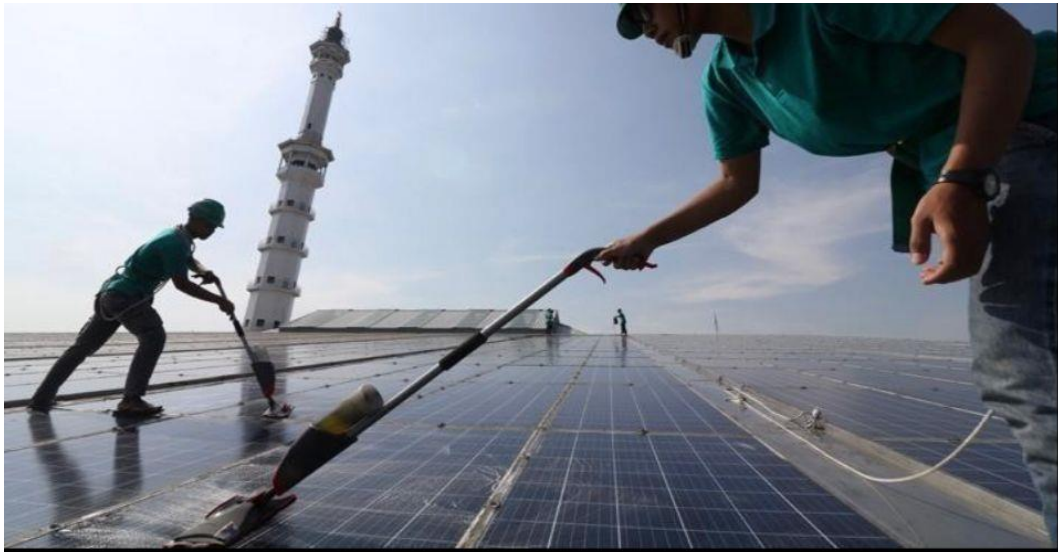
Gambar 2.3.13 Contoh Jasa Operation & Maintenance (Sumber: Data Internal PT Indosolar Energi Mandiri)
