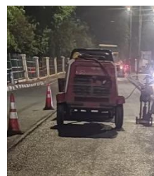
Gambar 3. 28 Air Compressor (Source: Dokumen Pribadi)
