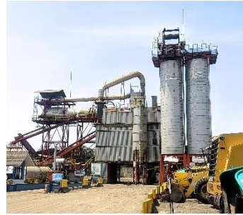
Gambar 3. 24 Asphalt Mixing Plant (Source: Dokumen Pribadi)
